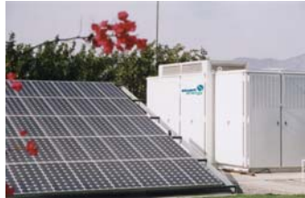
Solar & REC Electrolysis
